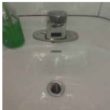
Sensor tape in factory toilet
